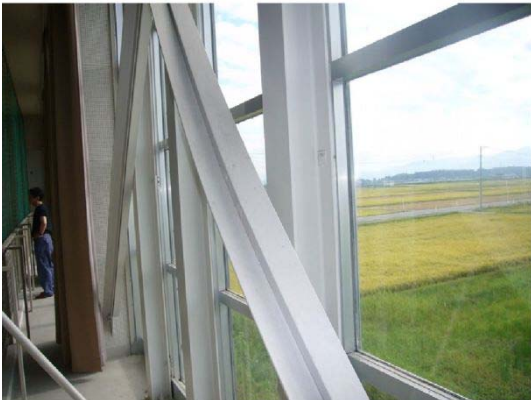
筋かい材の座屈 (刈羽村)
